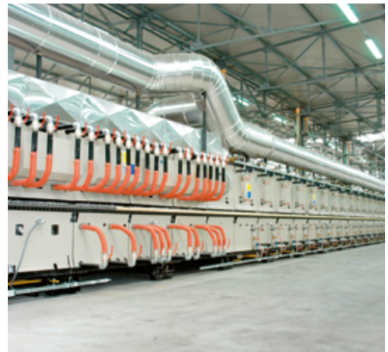
Roller hearth furnace
