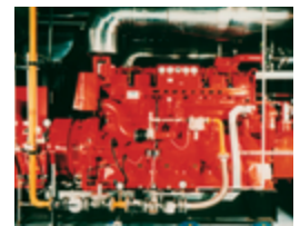
Stainless steel flexible tubes on gas engine sup- ply lines
