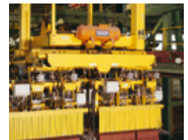
Stainless steel flexible tubes and bellows units at the kiln in the brick- works
