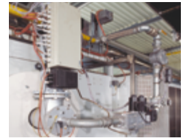
Stainless steel flexible tubes in the supply lines of buildings
